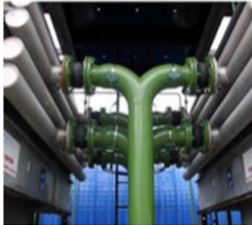
Central heating and air conditioning water
